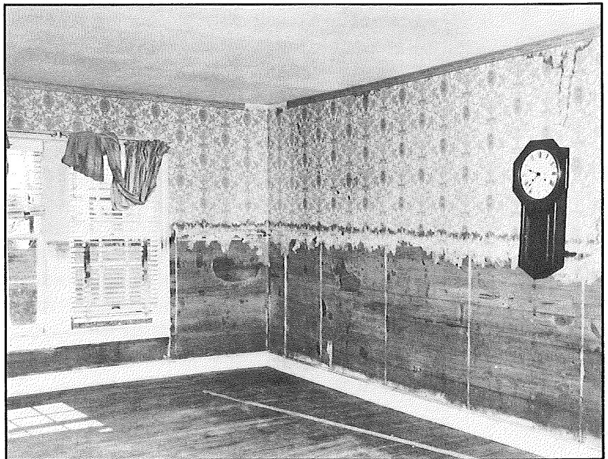
The water damage line in this Brownwood home bears silent but compelling witness to the awesomeness of Carla's flood tides.
